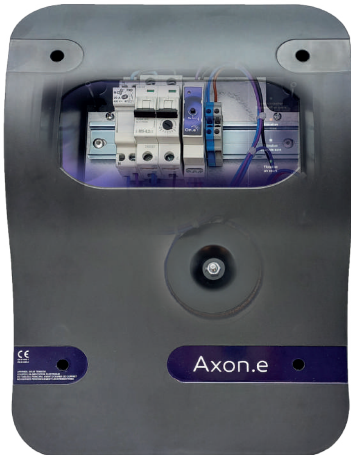
EXAMPLE OF A FILTER BOX (PRIVATE POOL)
